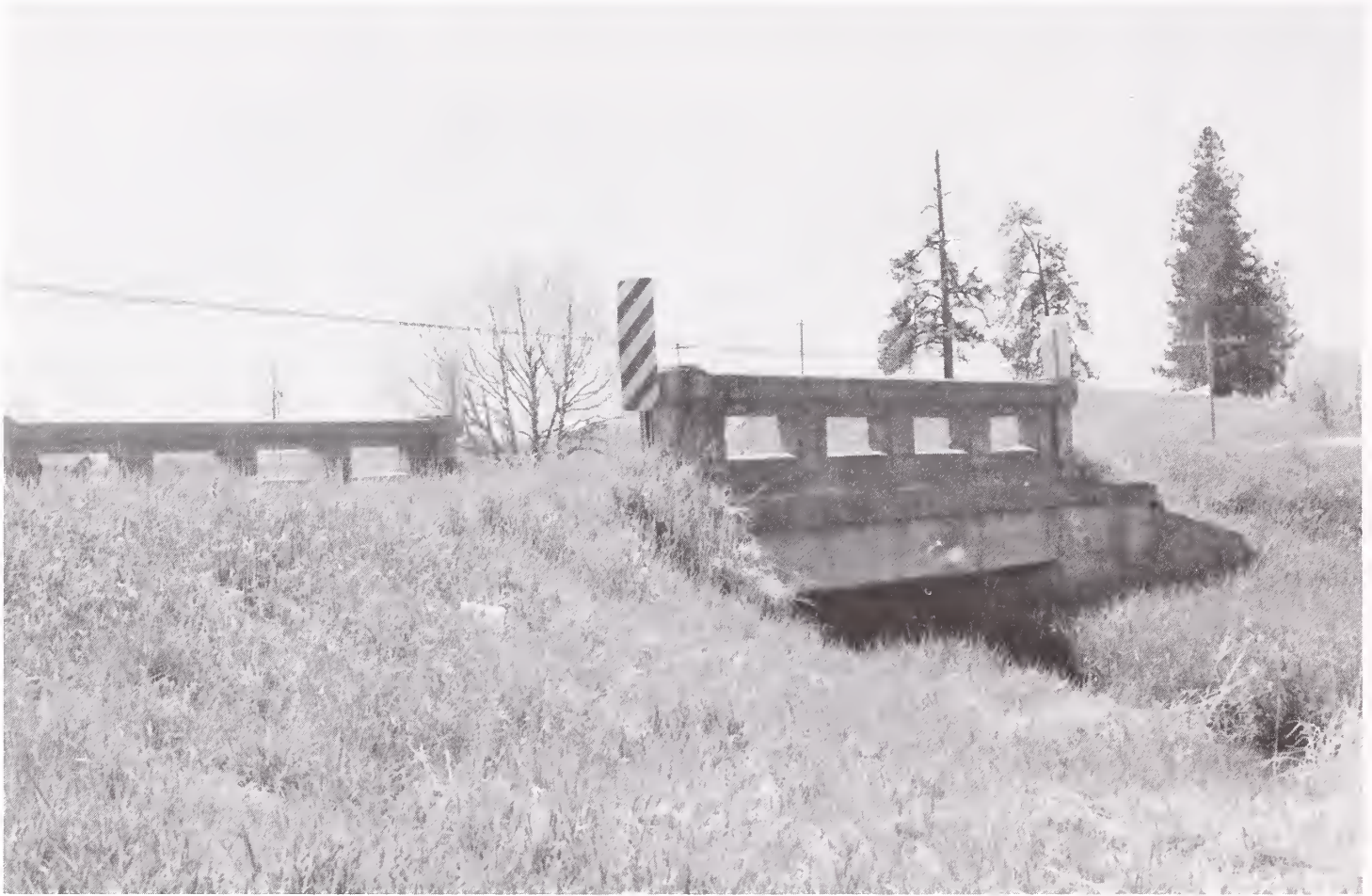
The Mud Creek Bridge was constructed shortly after the Bridge Bureau developed plans for the design.
